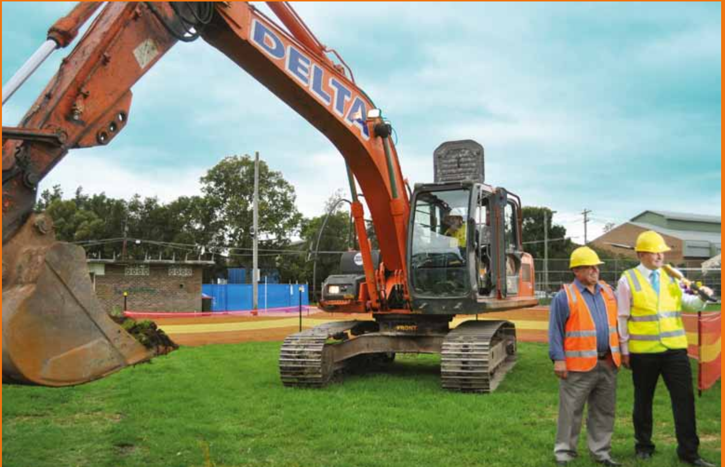
The Mayor of Marrickville Councillor Sam Iskandar and Member for Grayndler and Minister for Infrastructure Anthony Albanese turn the first sod to mark the commencement of work at Mackey Park earlier this year
